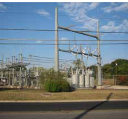
A transformer station in Northeast Austin.
