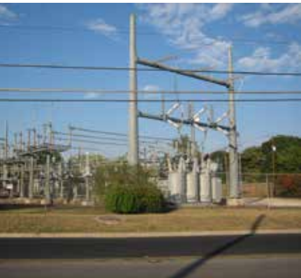
A transformer station in Northeast Austin.
